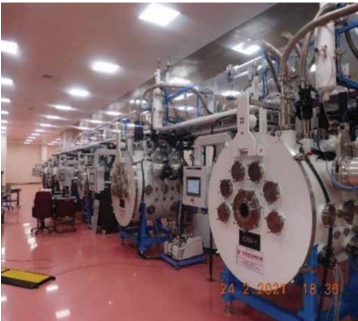
Installation, Commissioning & Operationalisation of 6 nos. of Thermal Vacuum chambers @ New Bopal Campus
