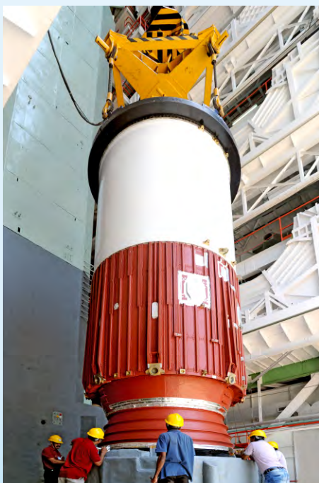
Placement of Base Shroud and Nozzle End Segment Module of PSLV-C38 core stage on the launch pedestal
