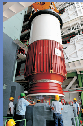
Nozzle End Segment of PSLV-C21 first stage being placed on launch pedestal
