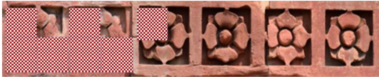
(b) Identifying broken area
