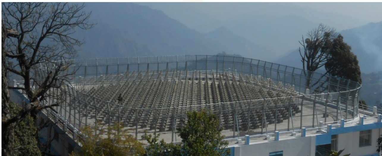
ST Radar antenna array on the roof-top of the building.
