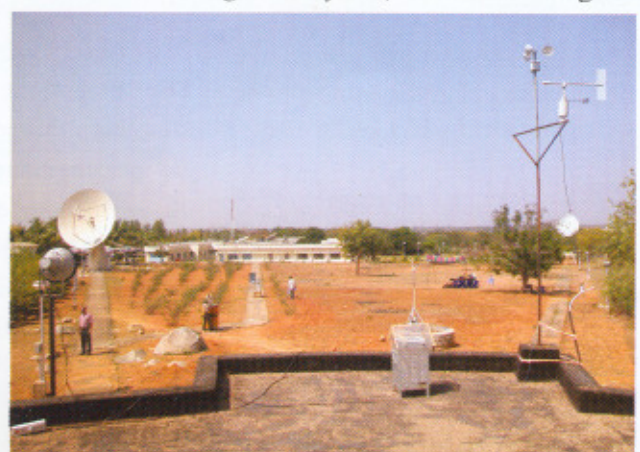
High volume air samplers & other meteorological instruments at Shadnagar
