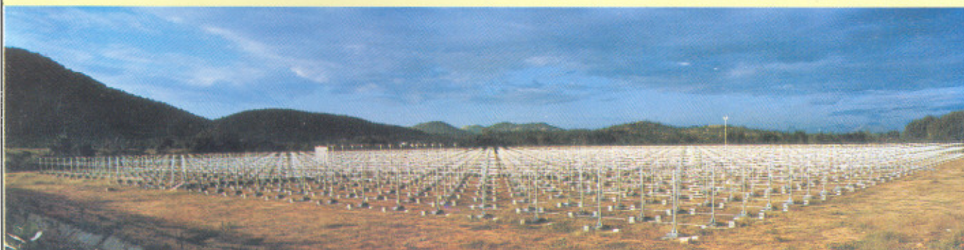
The Yagi antenna array of NMRF at Gadanki
