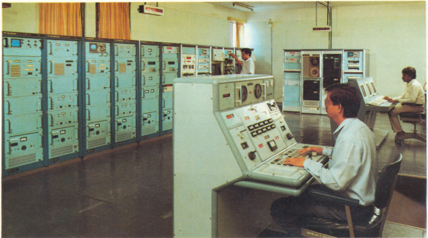
Telemetry station at SHAR
