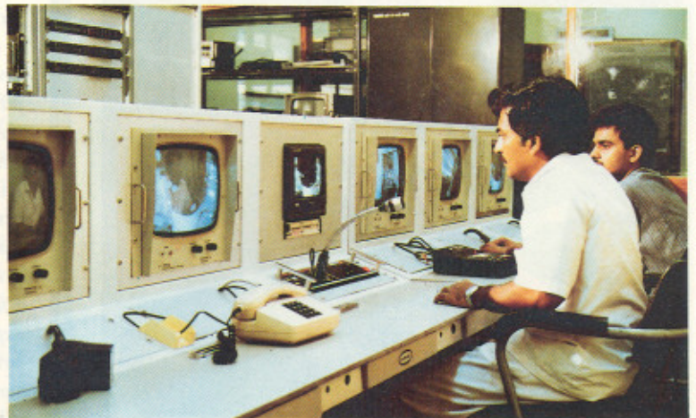
CCTV Control Room
