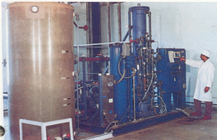
De-ionised water plant for cooling xenon lamps.
