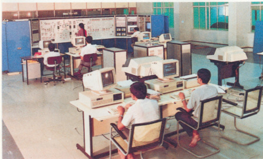
Central Control Console.
