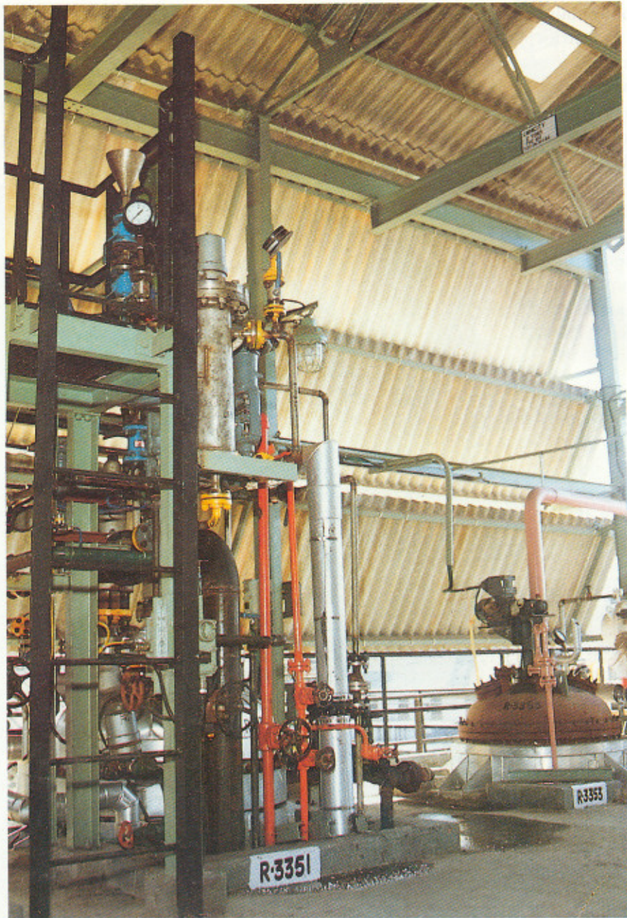
HTBP Plant at NOCIL based on ISRO technology.
