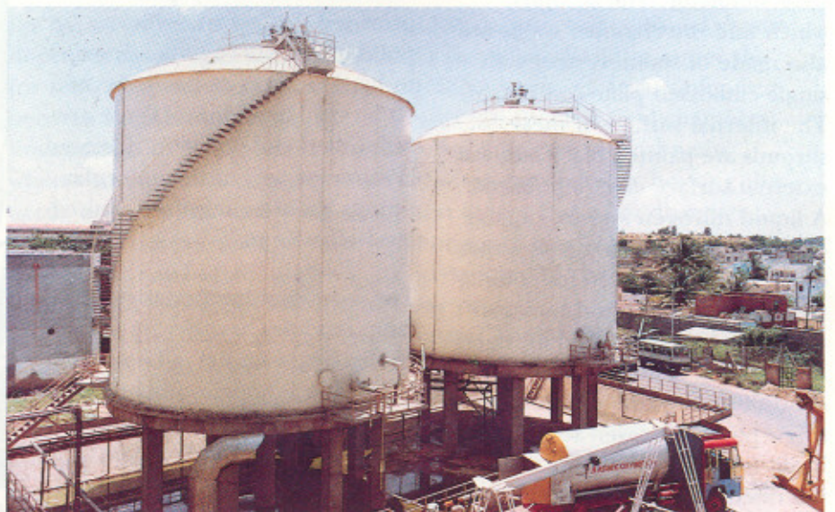
One million litre capacity liquid nitrogen tanks.
