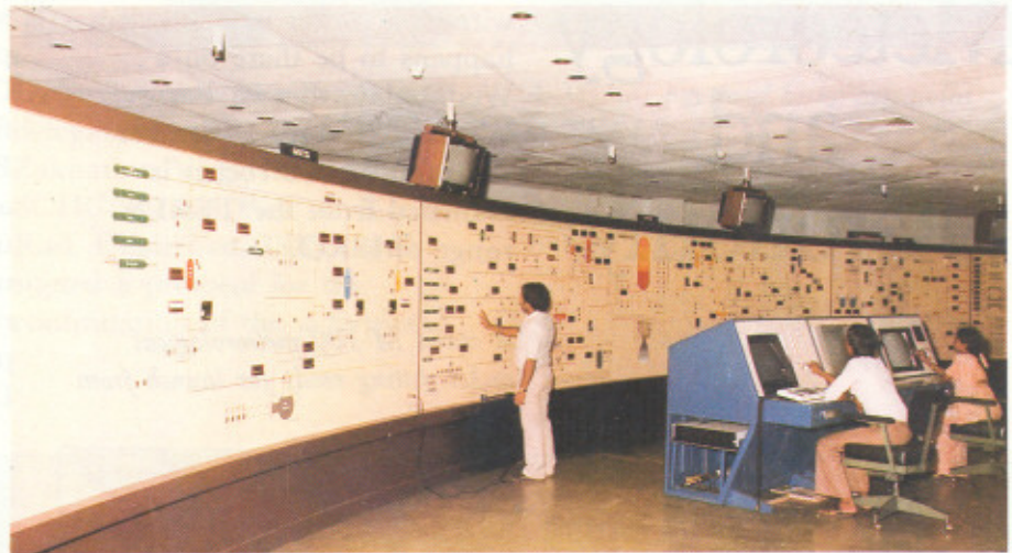
The Central data processing facility at LPTF, Mahendragiri
