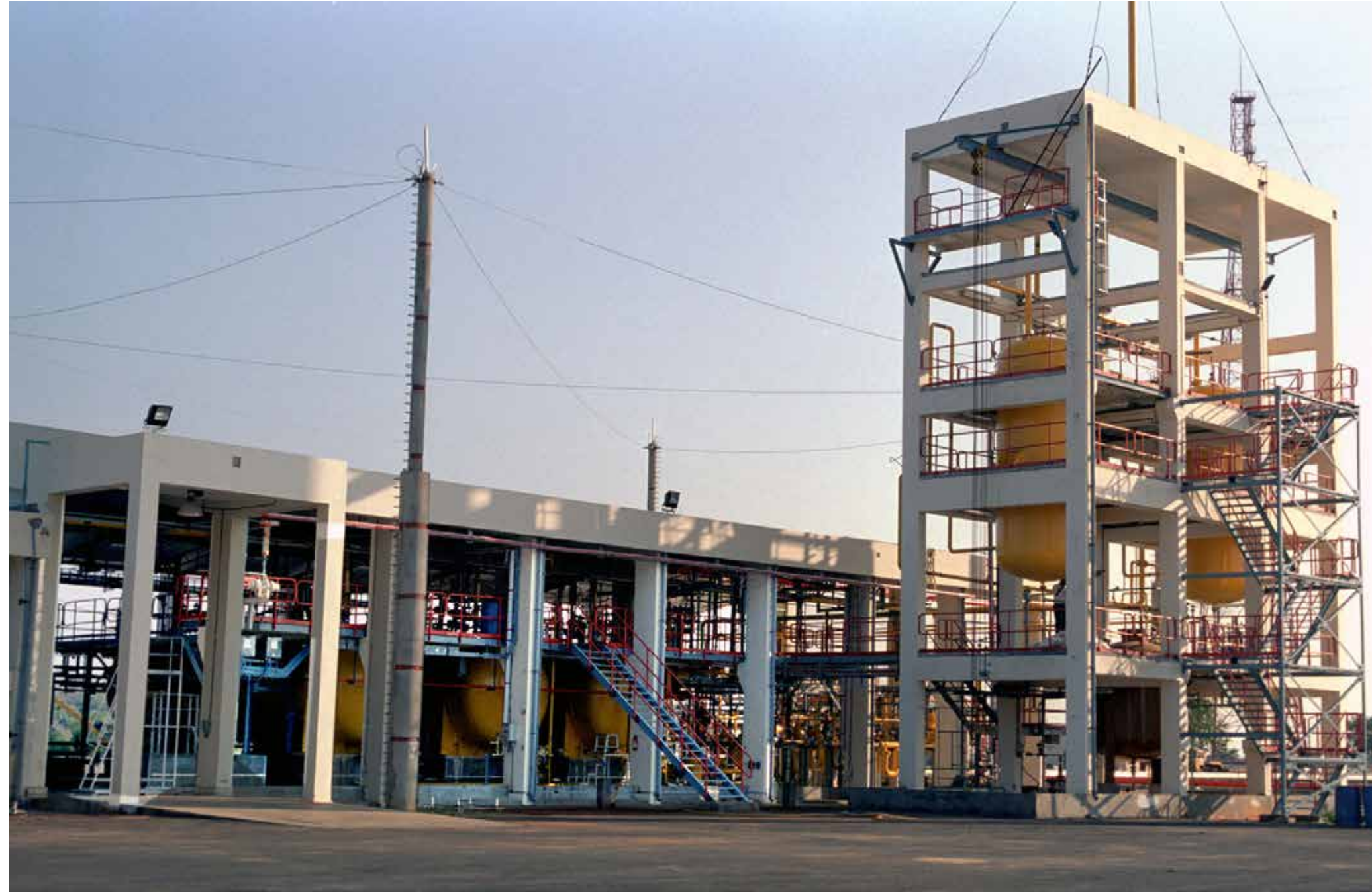
भंडारण सुविधा Storage Facility
